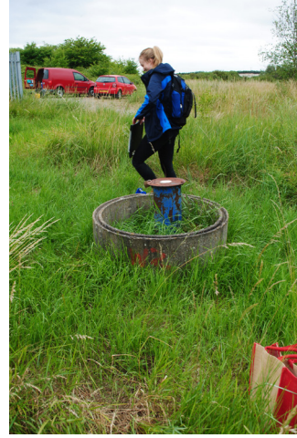
CMS monitoring well at leachate pumping station
